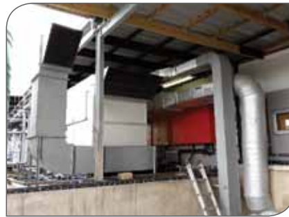
Main fresh-air AHU with crossflow heat recovery and supply air duct to kitchen makeup air.
